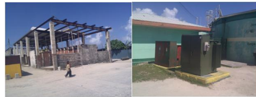
Figure 4: Photo of warehouse roof deterioration due to rust (left) and water plant next to electrical power station (right).
